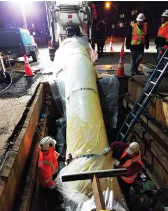
Starline® Cured in Place Liner coming off the drum guided as it enters the host pipe
