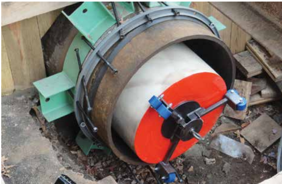
Custom pig fabricated to remove stranded grit
