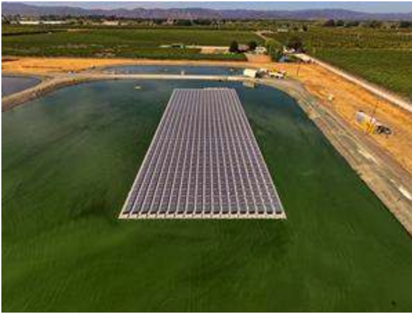
• The Ciel & Terre Hydrelío Floating Solar Power System installed at the Kelseyville County Waterworks, Dist. #3
