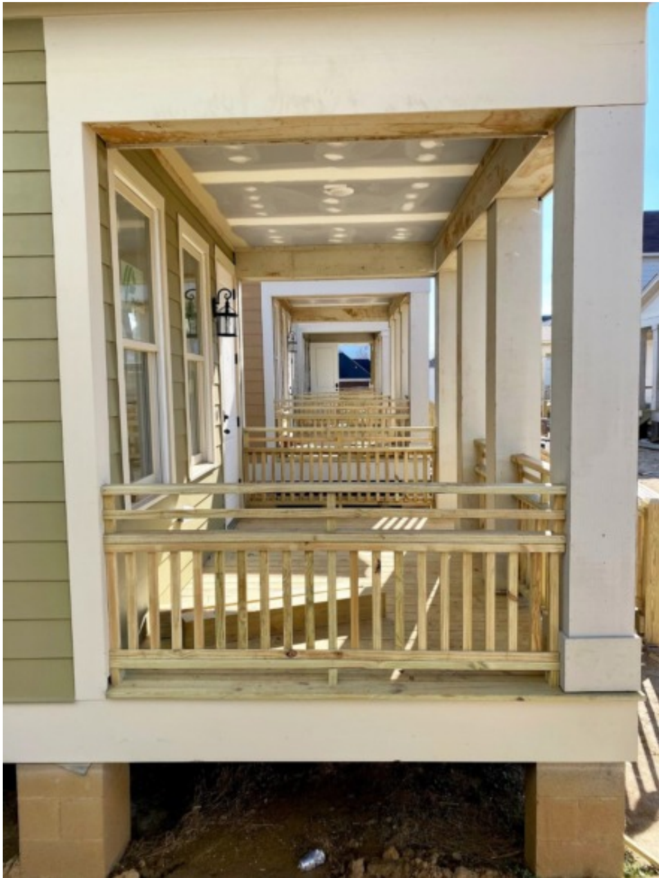
Porches provide space for chairs, tables and social interaction. Pier-and-beam foundations elevate the cottages and make maintenance easier. Latticework will soon cover the openings. (Tom Bailey/Daily Memphian)
