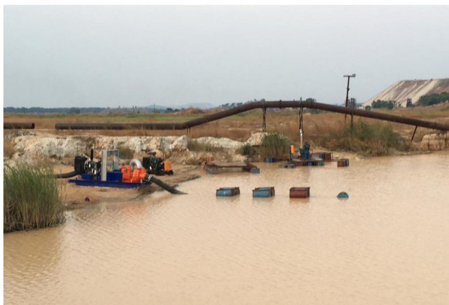
Figure 2. Pumping operations at the NE end of Roche Dure near the historical sump pump
