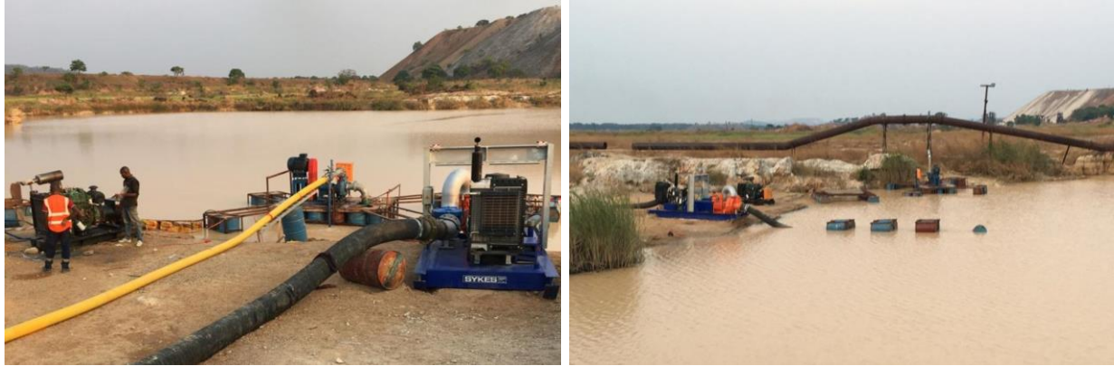
Figure 1 & 2. Sykes pump to right and spindle pump on the pontoon operating at the NE end of Roche Dure near the historical sump pump
