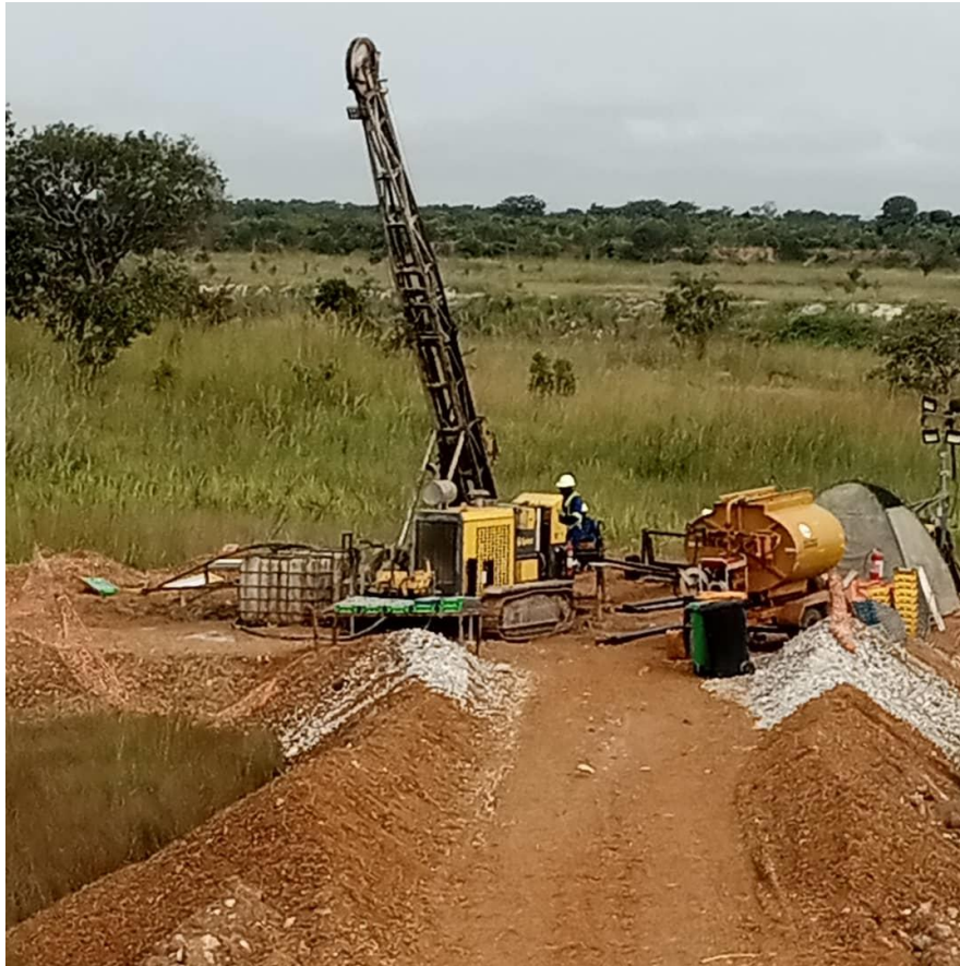
Figure 7: Drilling on causeway built over marshy ground. Roche Dure pit in background
