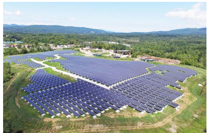
Solar panels, Sterling, MA
