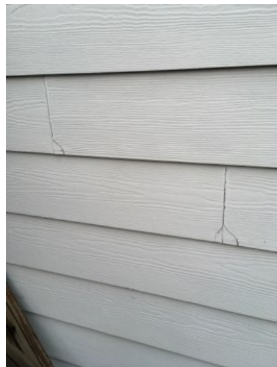
Cracked siding on left side of the house.
