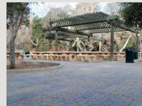
Permeable pavers at Oak Park were installed by the City to help reduce polluted runoff.
