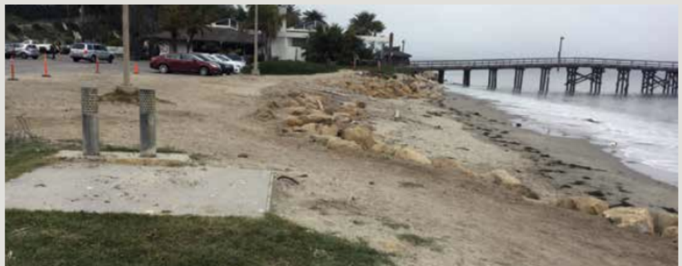
The GSD Vault (lower left square metal top), houses the infrastructure connecting wastewater plant and ocean outfall. It sits at the edge of Goleta Beach, which is eroding rapidly. (Hillary Hauser photo)
