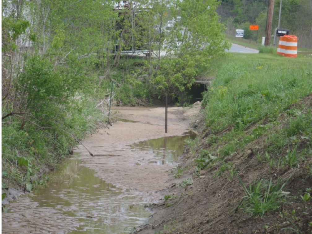
Figure 14. Sedimentation in Walker Ditch.
