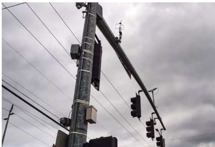
Figure 10: The traffic signal pole and mast arm equipped with a 3D sonic anemometer for wind speed and direction, temperature and relative humidity probe, and cameras and radar for traffic counts on the SW corner of the intersection of SE 122nd Ave and SE Division St.
