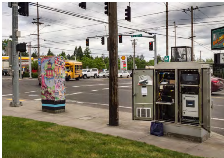
Figure 9: The City of Portland Curbside Lab for Emissions and Atmospheric Research cabinet on the right at the intersection of SE 122nd Ave and SE Division St. The traffic signal cabinet operating the signals and decorated with community art is on the left
