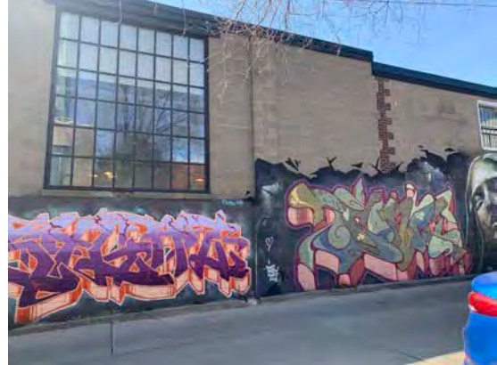
North elevation of 376R Dufferin Street (left) where it meets 358 Dufferin Street (right) along Milky Way Lane.
