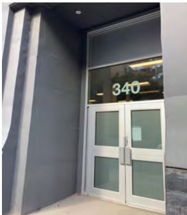
Non-original door opening at 340 Dufferin east elevation (ERA, 2021).
