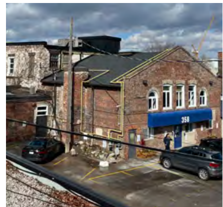
South and east elevations of the core oven building from the interior courtyard.
