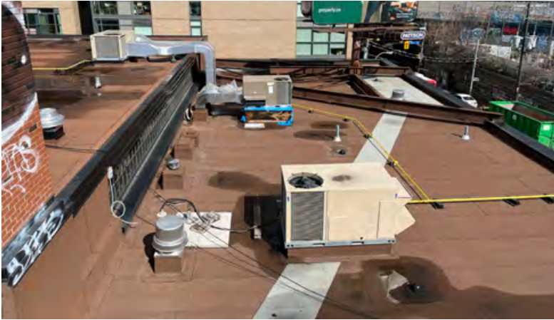
Roof condition at 366-370 Dufferin Street (ERA, 2022).
