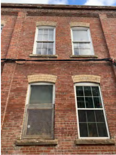
Typical bay along the south elevation with a mix of wood and vinyl windows (ERA, 2021).
