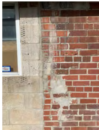
Unsympathetic concrete block infill around the main entrance to 358 Dufferin St. (ERA, 2021).
