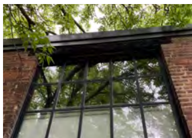
New windows and flashing and original wood lintel at 358 Dufferin Street (ERA, 2021).
