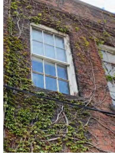
Vine growth along west elevation. Original wood window with a 6-over-6 pattern (ERA, 2021).
