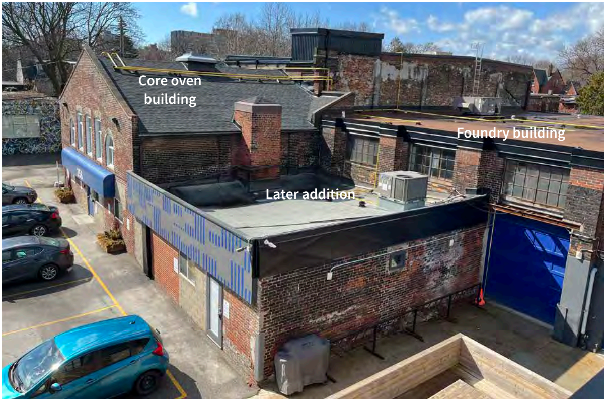
North (and partial east) elevation of 350 (left) and 358 (right) Dufferin Street. Note: March 2022.
