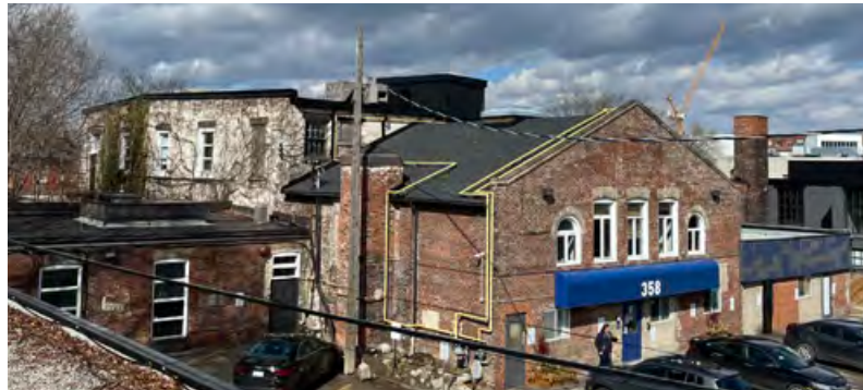
Varied functional building forms, including the mixing building and core oven building at 350 Dufferin Street (more intact) and the foundry building at 358 Dufferin Street (less intact due to loss of gabled roof). The address of the east elevation onto the central courtyard (March, 2022).
