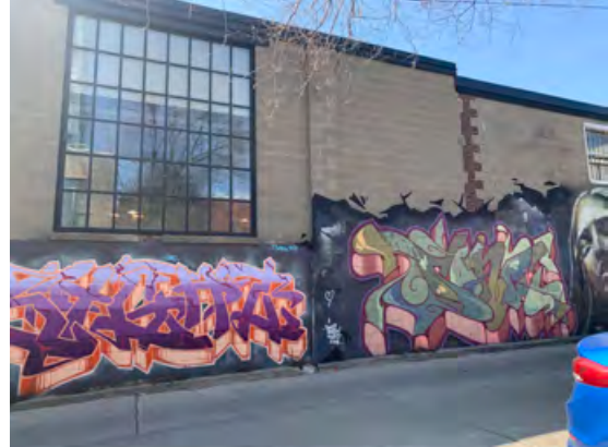
North elevation of 376R Dufferin Street (left) where it meets 358 Dufferin Street (right) along Milky Way Lane.
