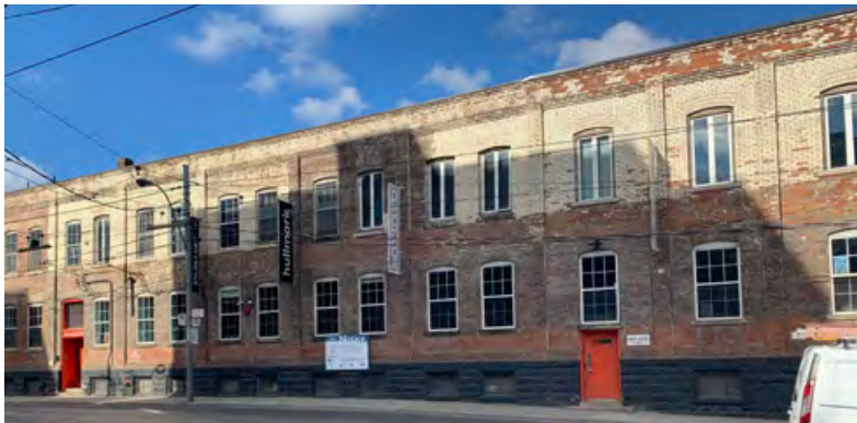
360 Dufferin St. east elevation showing masonry elevations with corbelling, flaking paint along the facade, select window replacements, painted stone water table (ERA, 2021).
