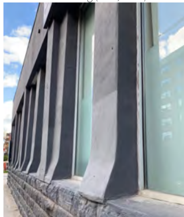
East elevation of single-storey building with altered window openings and parging (ERA, 2021).
