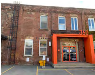
West elevation: new metal ladder and entrance canopy. Select infill of windows (ERA, 2021).
