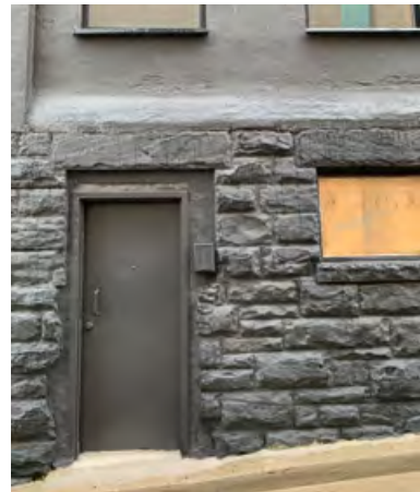
Altered door opening and boarded window at 366-370 Dufferin Street (ERA, 2021).
