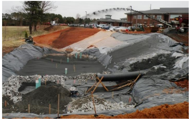
Figure 14 Installation of Bioretention Cell at the Hospice of Wake County- Raleigh, NC (March 2010)
