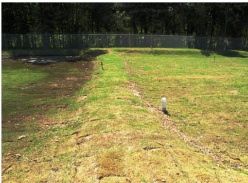
Figure 12 Post Installation Photo of Bioretention Cell at North Mecklenburg Solid Waste Recycling Center - Huntersville, NC (August 2009)
