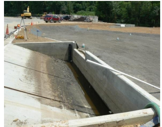
Figure 10 Installation of Bioretention Cells at North Mecklenburg Solid Waste Recycling Center - Huntersville, NC (July 2009)
