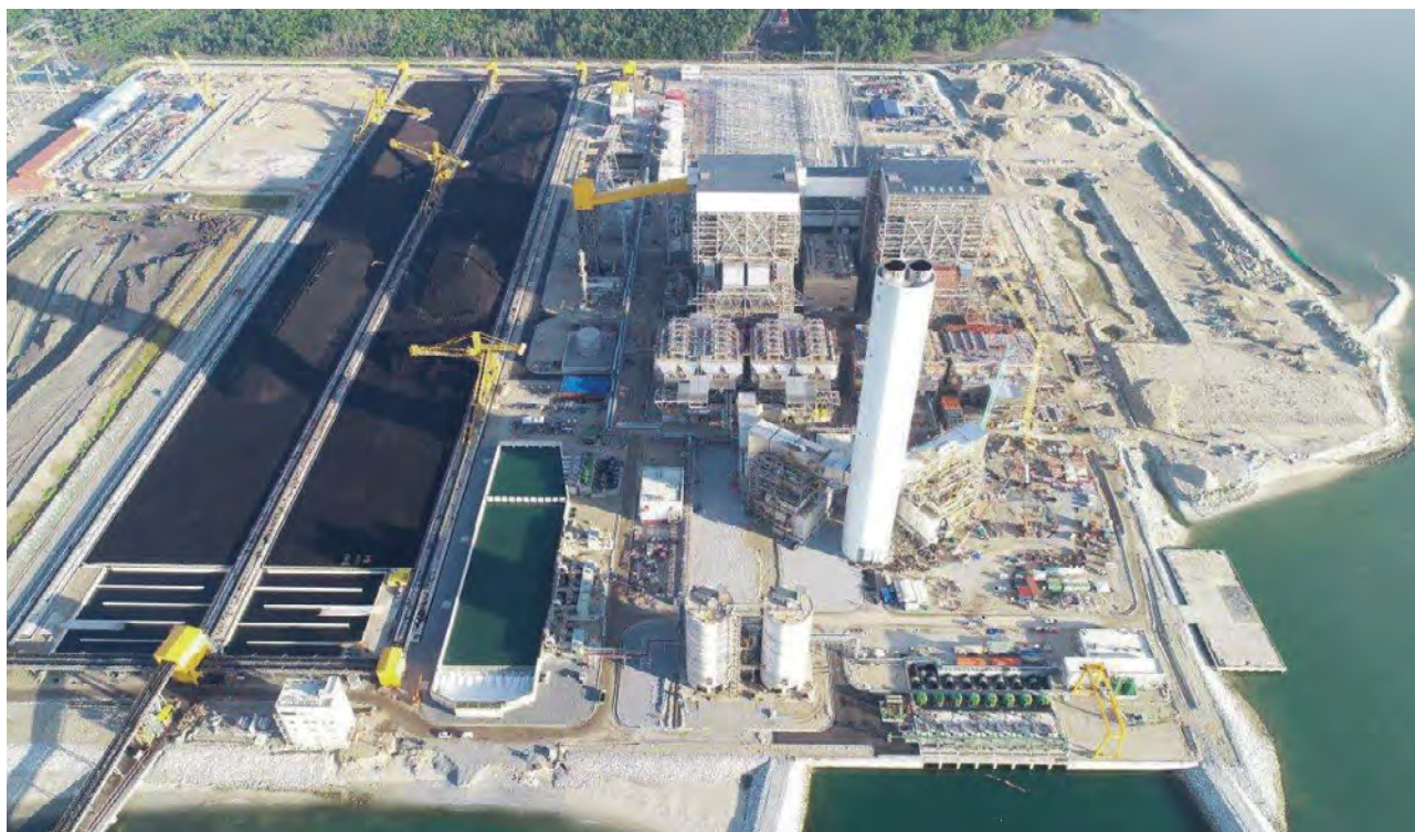
Jimah East Coal-fired Power Plant in Negeri Sembilan, Malaysia (Chugoku Electric Power Co., TNB, and Mitsui & Co.) Jimah East is a USC plant with an output of 2,000 MW (1,000 MW × 2 units). Commercial operation started in 2019.
