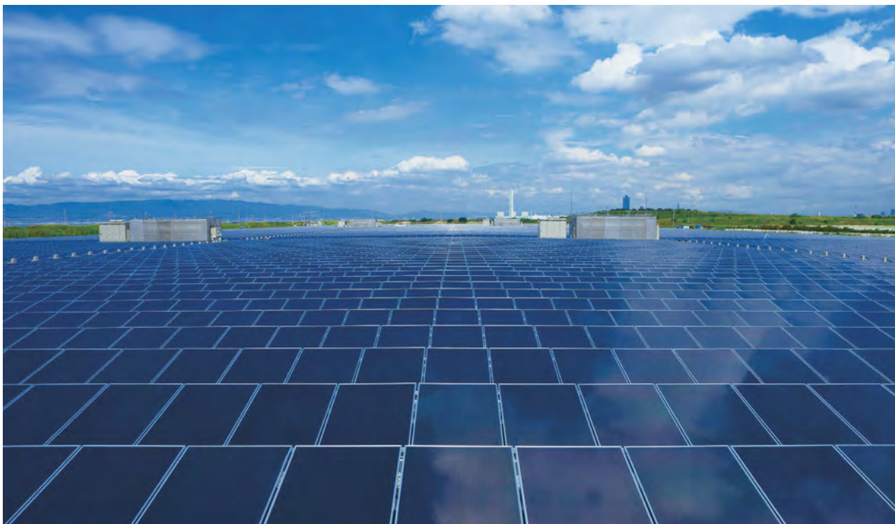
Sakai Solar Power Station (Kansai Electric Power Co.)
