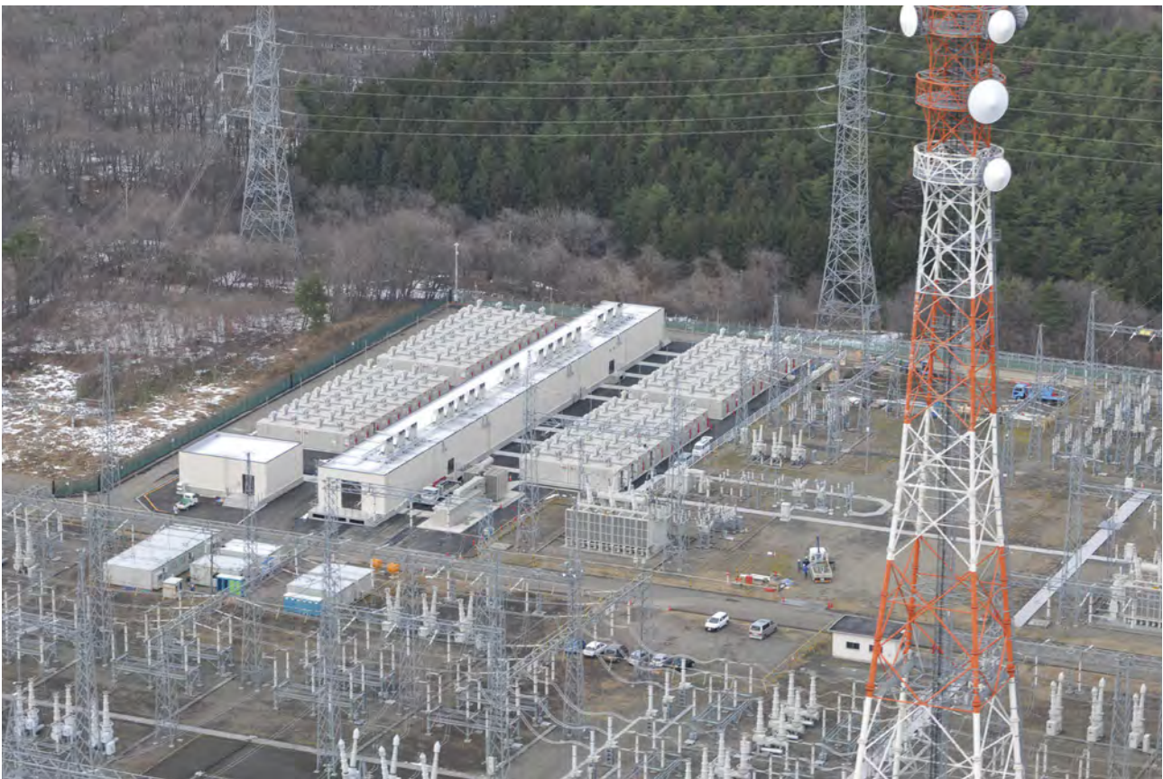
Nishi-Sendai Substation Storage Battery System (Tohoku Electric Power Co.)
