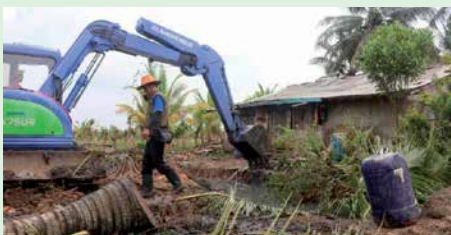
Tree trunk etc which allowed backhoe access to project site bridge unsafe to cross – Degraded
