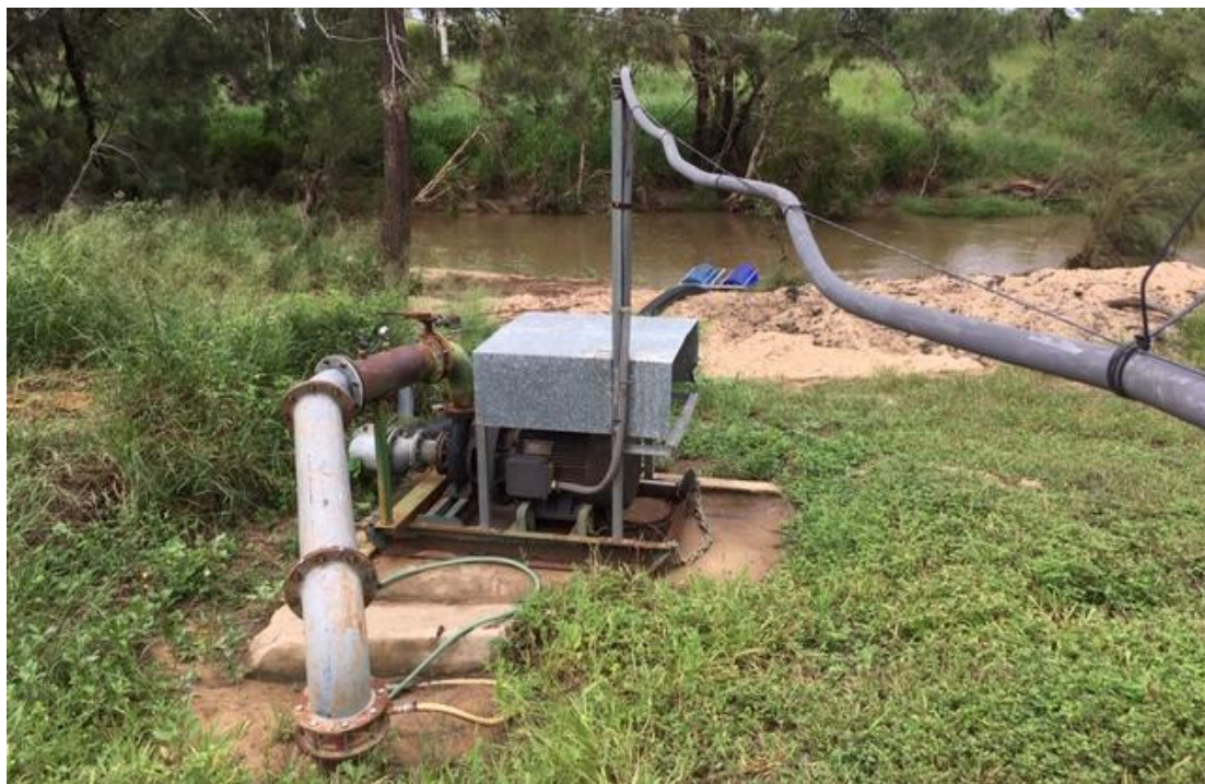
Figure 13: 55kW grid-connected pump in the Tablelands.
