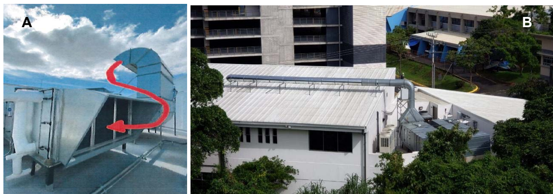
Figure 1. A. Inlet and outlet pipe HVAC system initial arrangement installed in the building and radioactive gas trajectory entering production main floor. B. Final placement of the outlet pipe.
