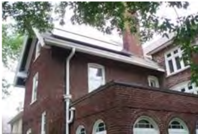
Solar installation on an historic building in Michigan. 35
