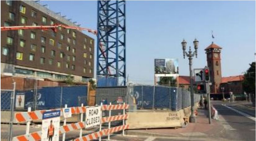
New high-density development, such as the Bud Clark Commons (left) and Multnomah County Health Department facility (under construction), are altering the once utilitarian transportation land uses in the vicinity of Union Station.
