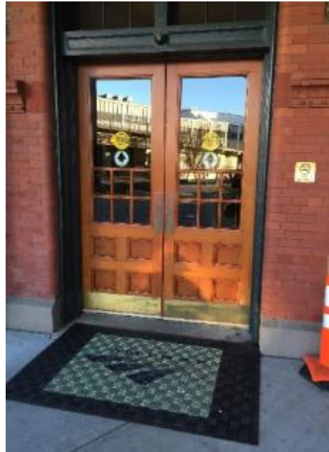
Power-assisted station entrance door
