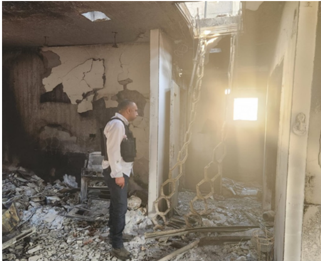
Rev. El Shafie surveys the ruins of a home destroyed by Hamas terrorists in the attack of October 7, 2023.
