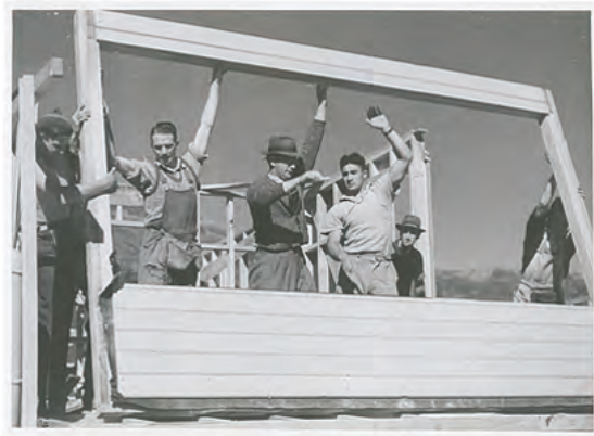
State housing panel programme utilising low skilled workers and panel based prefab construction.
