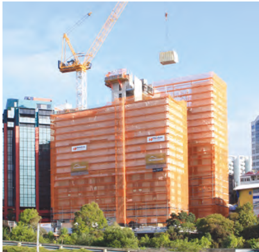
Stanley Group delivered over 400 bedsit modules to create University of Auckland's Student Accommodation Project, 2011.
