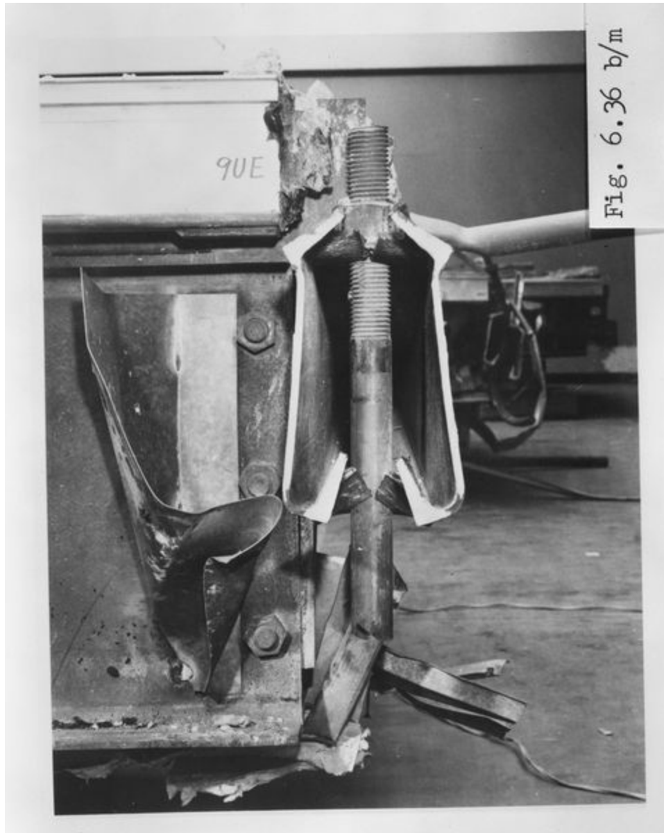
A front view of a beam section from one of the collapsed walkways. Department of Commerce. National Bureau of Standards/National Archives
