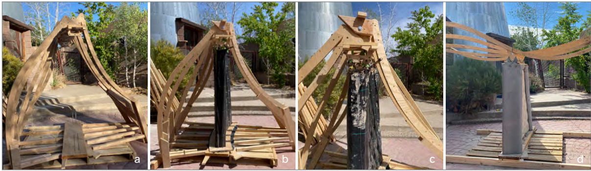
Figure 2. System timelapse showing the roof rafters as temporary support before final rotation.
