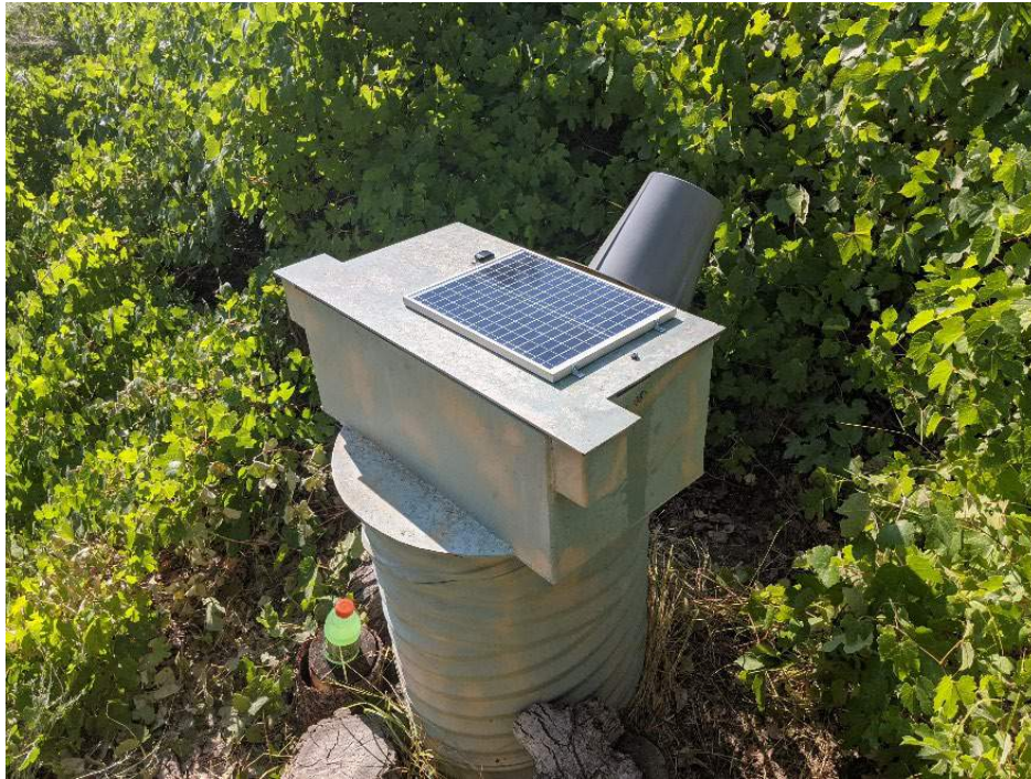
FIGURE 4. STILLING WELL AND ENCLOSURE WITH MOUNTED SOLAR PANEL AND SATELLITE ANTENNA
