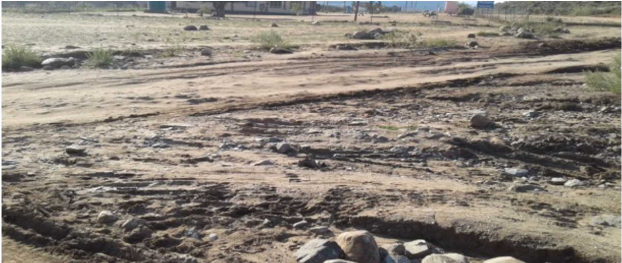
Morapaneng village access road in a bad state
