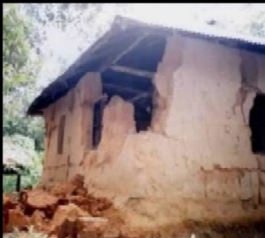
fig:6 one of the mud houses that collapsed due to rain.
