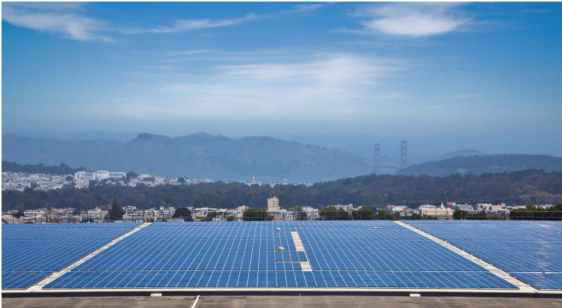
Photo 10: Sunset Reservoir Solar Panels (a CleanPowerSF source of power supply)
