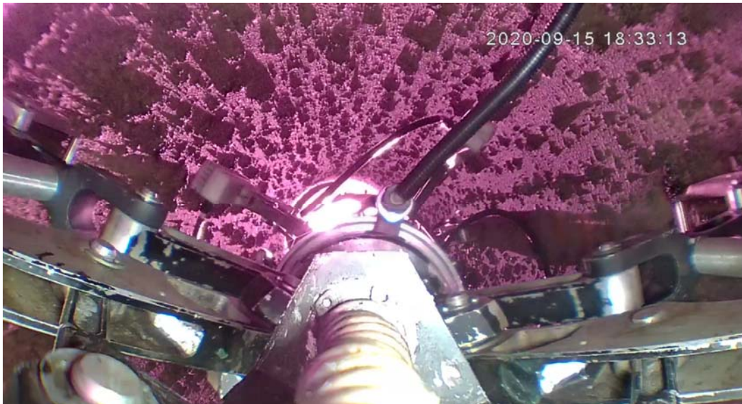
Figure 5: Tuberculation as see from Crawler Camera 3
