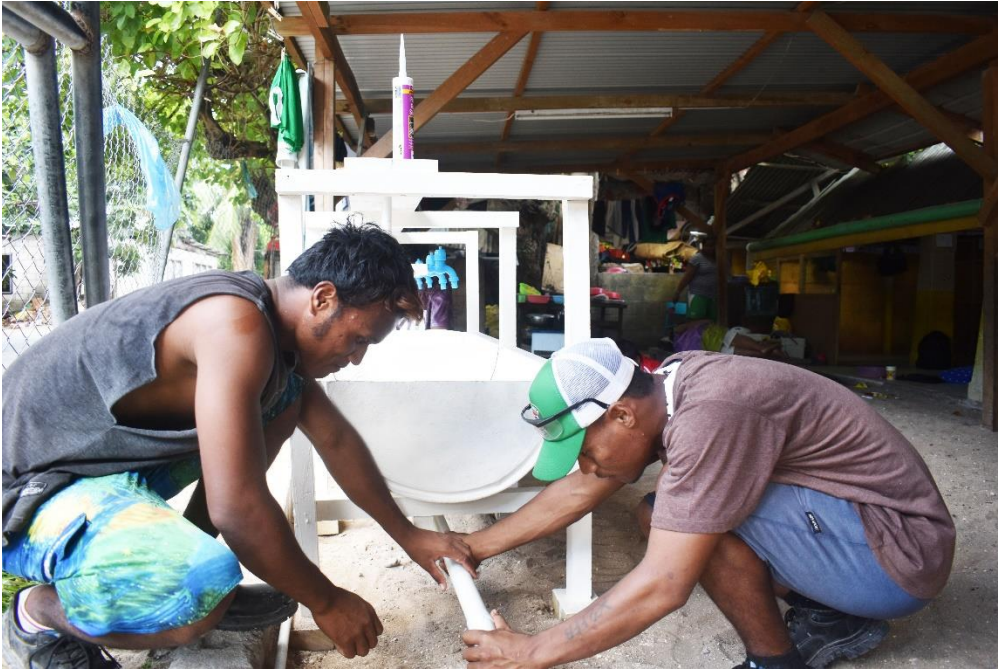
Photo: Locally-constructed handwashing stations in Kiribati used in the AHP COVID-19 response. The handwashing stations were positioned in community centres, and constructed by youth groups and Kiribati Institute of Technology students. Credit: Childfund Kiribati
