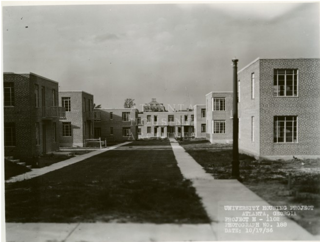
University Homes two-story apartment type under construction, Atlanta, GA, 1936. University Homes Records, photograph UNIV2013_img_01665 (Atlanta, Georgia: Atlanta Housing Archives, The Housing Authority of the City of Atlanta).
