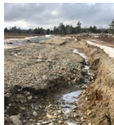
Washout on Cousins Road in 2019. (Photo: GPA)
