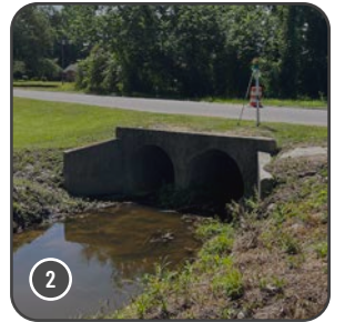
Williamson Street: Existing Culvert Condition
