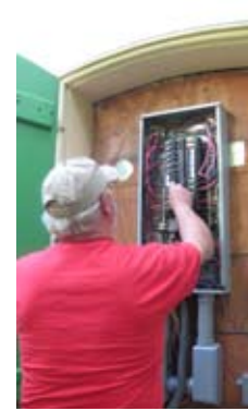
Left to right: old electric panels; Webb Johnson of Aurora Services
