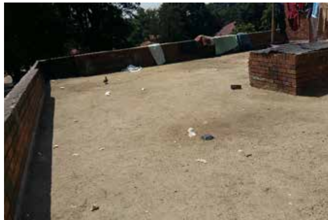
Figure 2c: Image of flat concrete roof. Waterproofing was removed between 2001-2003.
