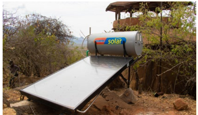
The borehole and Tassia Lodge were equipped with a solar power system.
