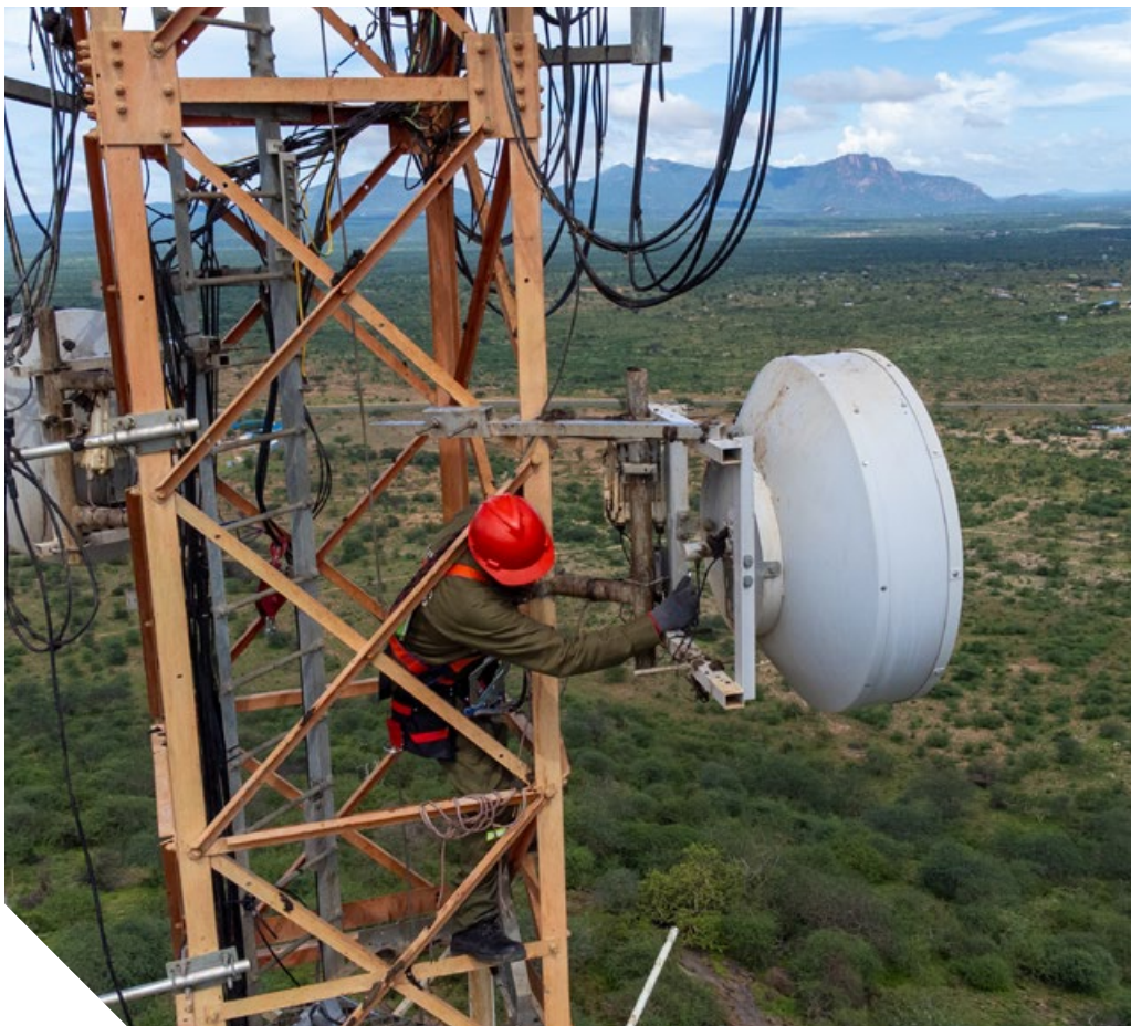
Security network installation in Kalama Community Conservancy.
