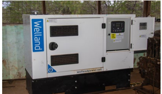
Purchased a generator to facilitate the pumping of water from the Ewaso River to the Biliqo community.
