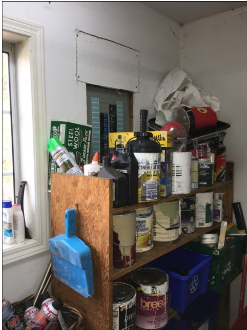
8.2 Item 1(Picture) Obstructed access.
