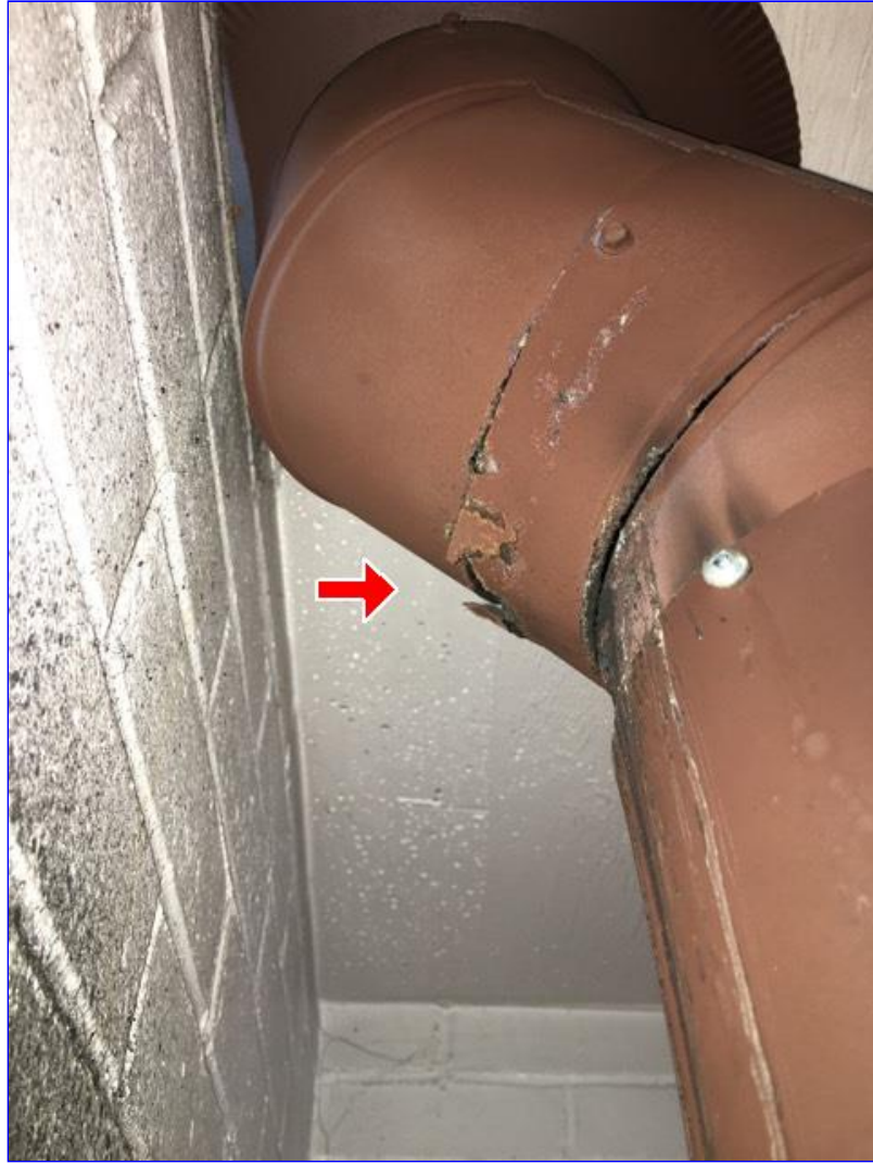
9.14 Item 1(Picture) Rusted out.
