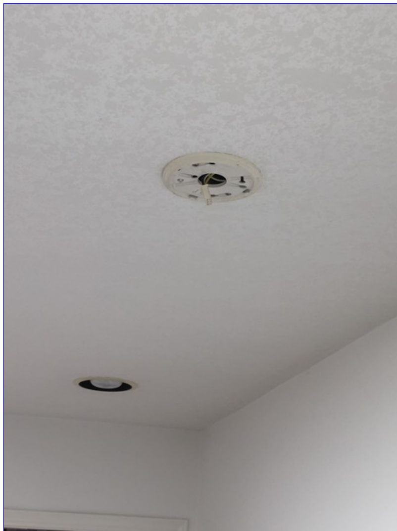
8.9 Item 1(Picture) Missing detector
