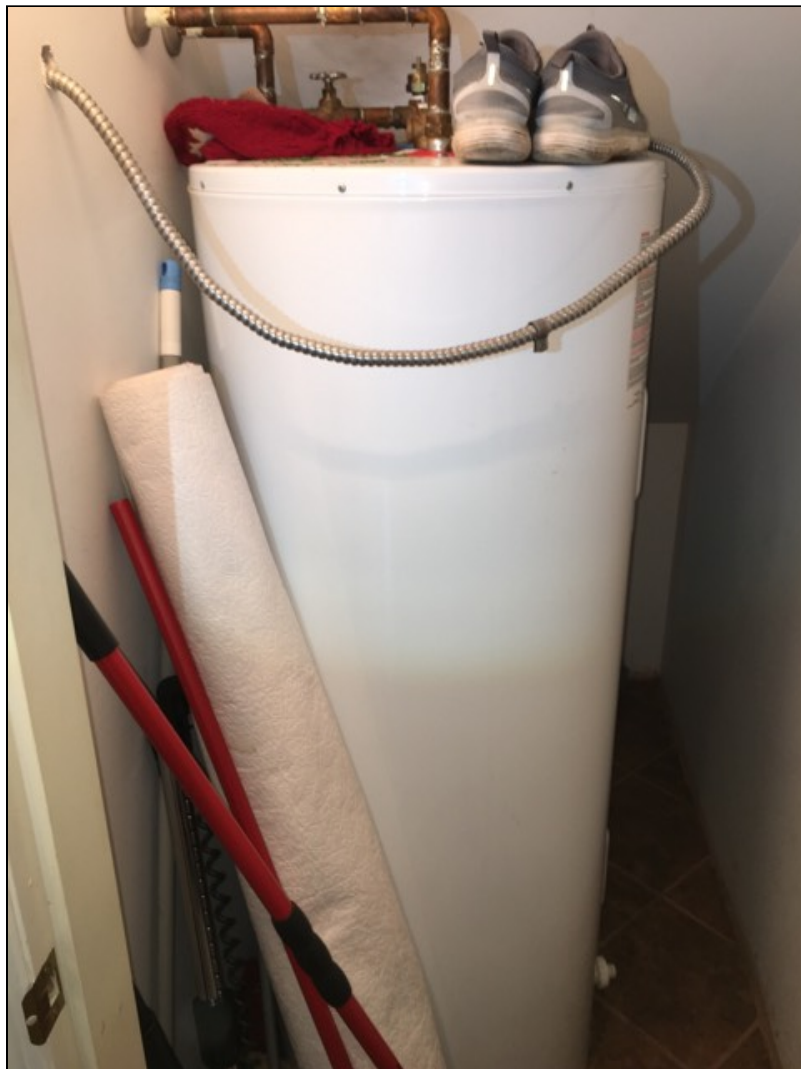
7.4 Item 2(Picture) No earthquake strapping
