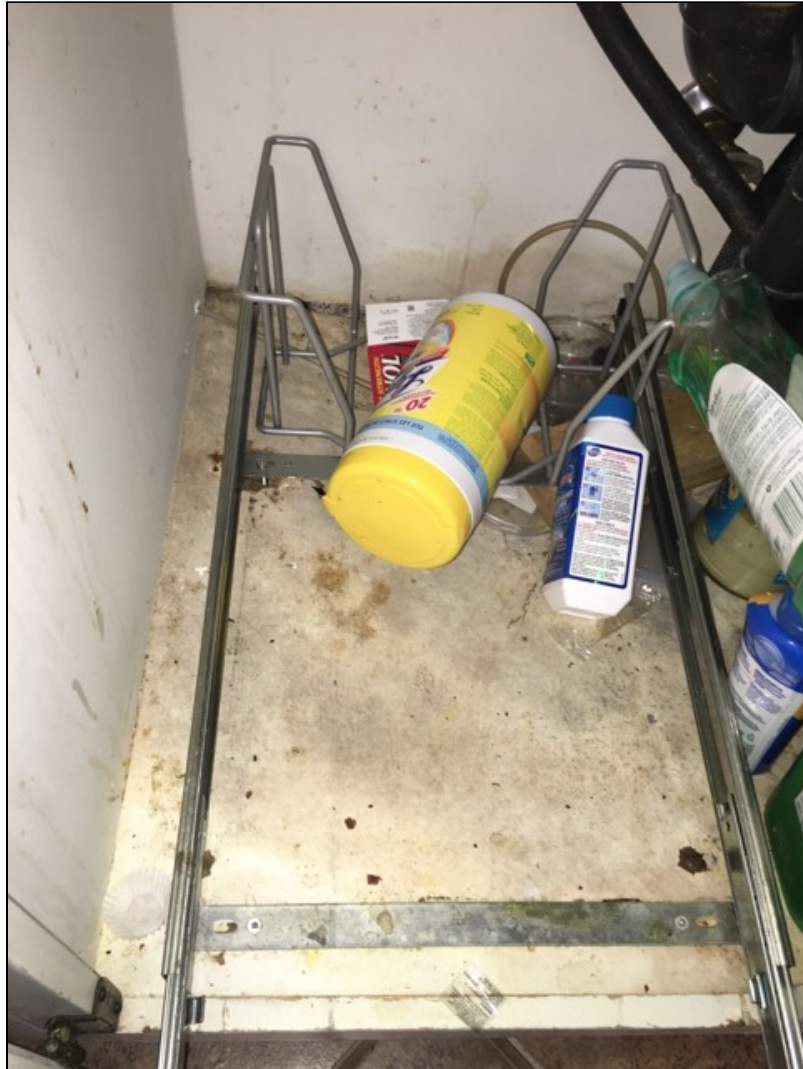
12.8 Item 1(Picture) Some damage from previous moisture
