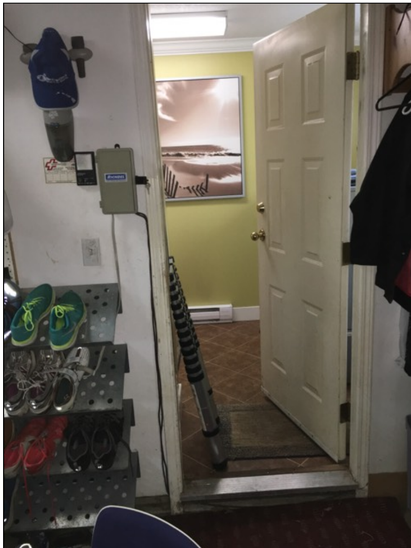
4.8 Item 1(Picture) Door does not automatically close and seal.
