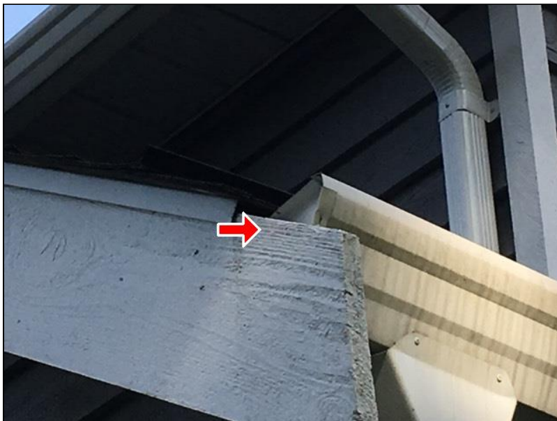
2.2 Item 1(Picture) Fascia boards exposed
