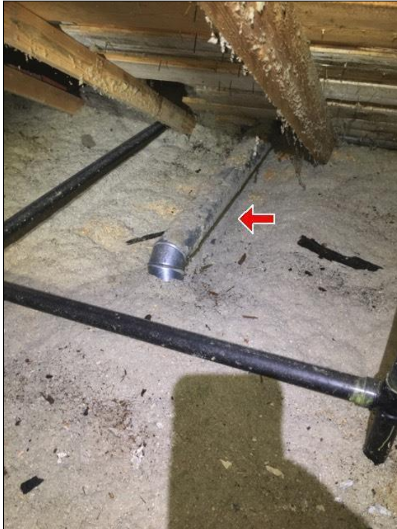
6.7 Item 1(Picture) Main bath vent duct
