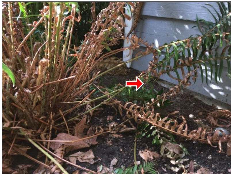
3.0 Item 1(Picture) Less than 6 inches to wood siding
