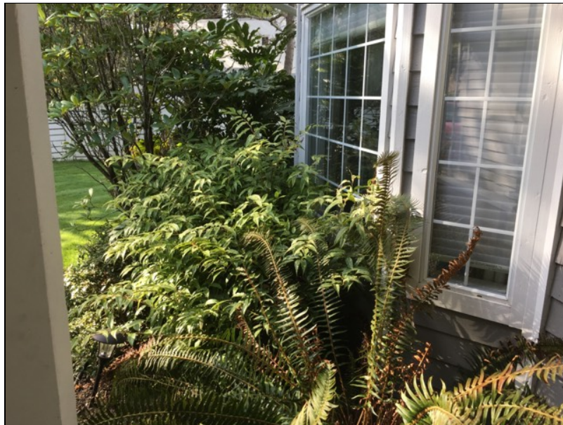
1.1 Item 1(Picture) Shrubs too close to building
