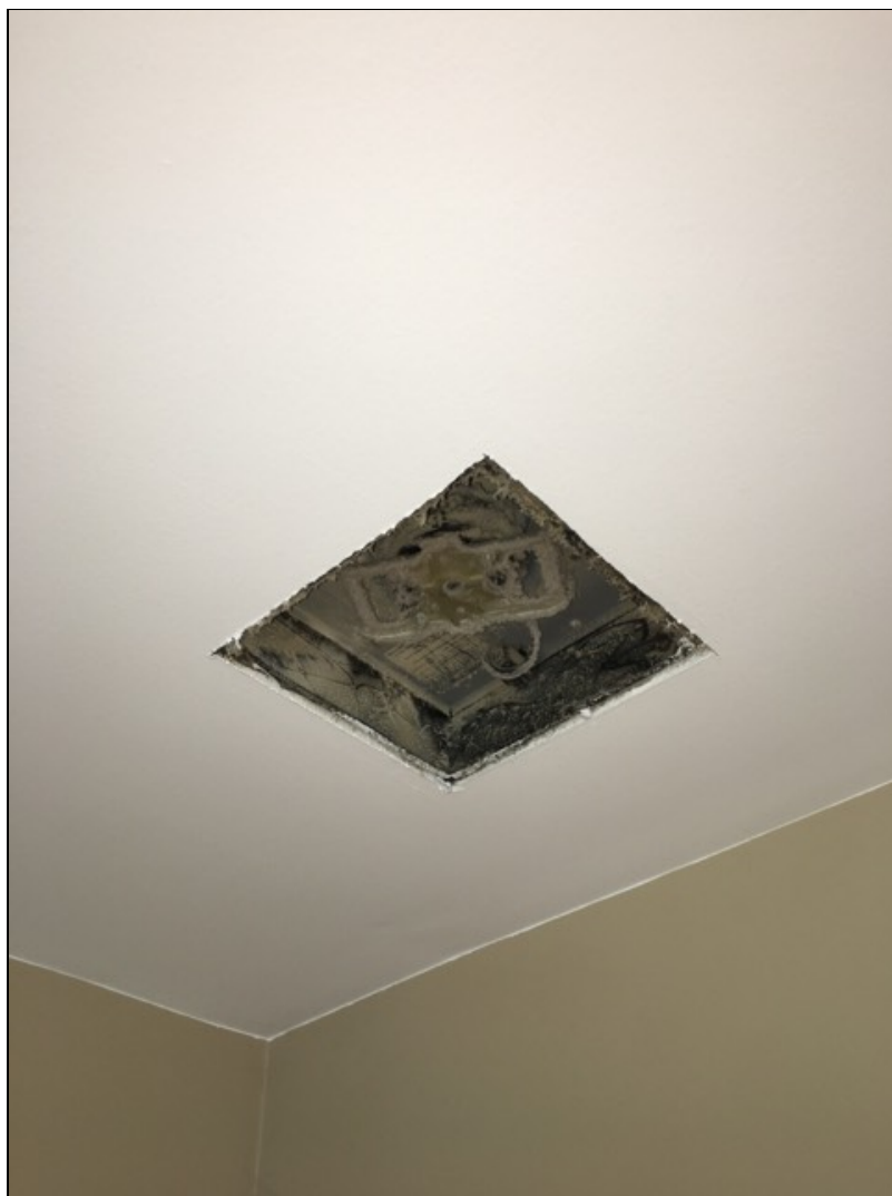
10.7 Item 1(Picture) Main bath fan
