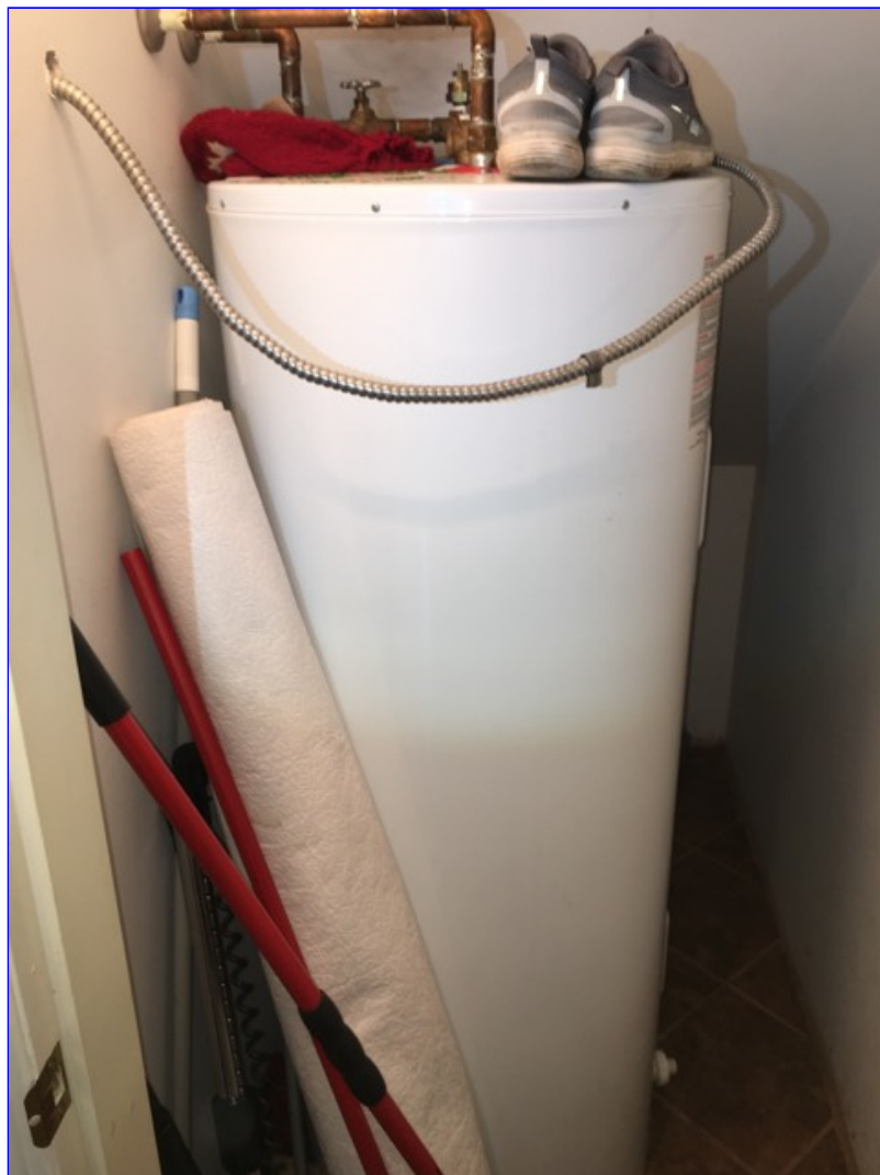
7.4 Item 2(Picture) No earthquake strapping
