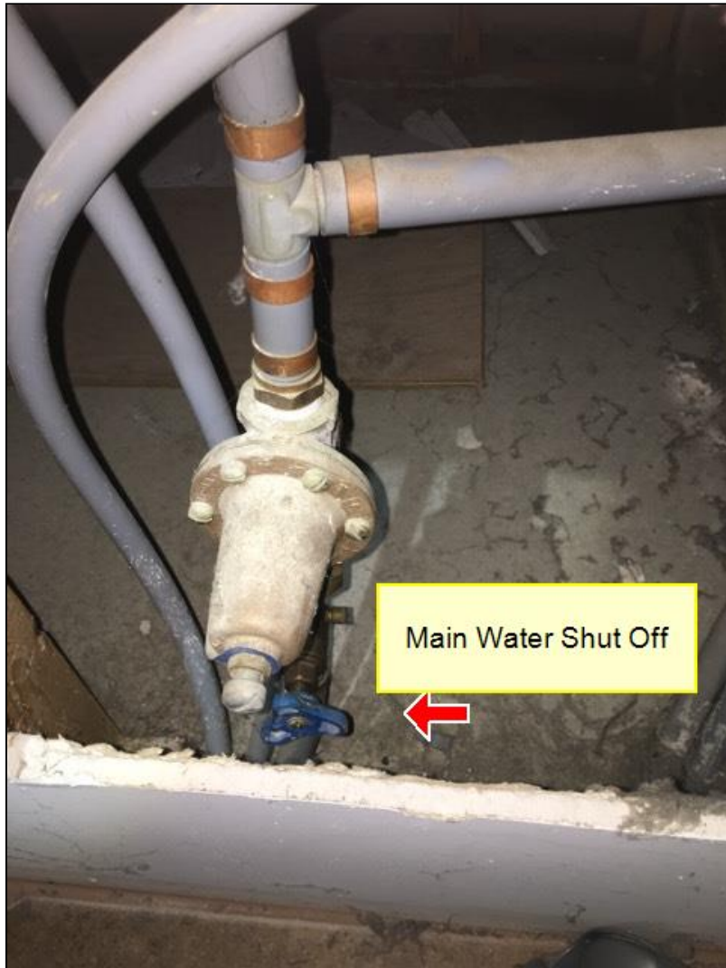
7.0 Item 1(Picture) Main shut off
