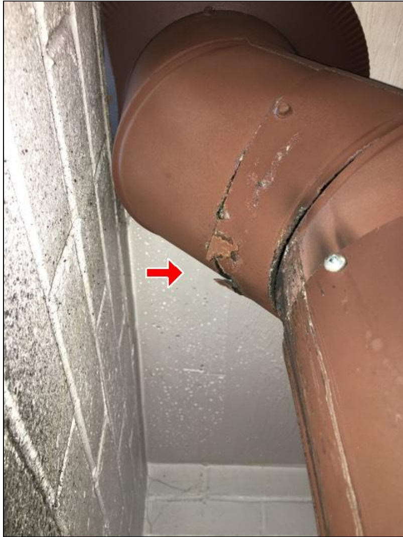
9.14 Item 1(Picture) Rusted out.
