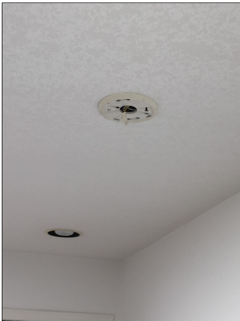
8.9 Item 1(Picture) Missing detector
