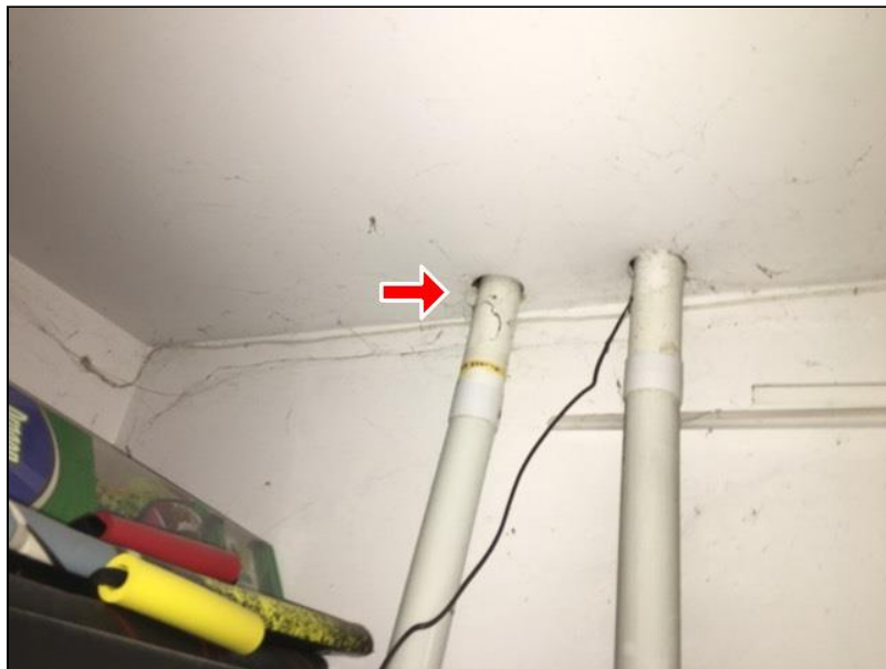
4.5 Item 2(Picture) Gap in drywall.
