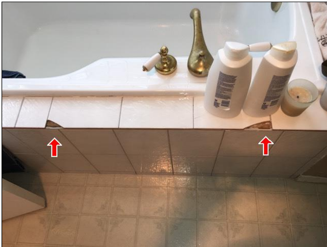
10.13 Item 1(Picture) Broken tiles
