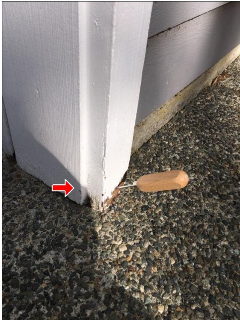
3.0 Item 2(Picture) Some rot noted at ground/wood junctions.
