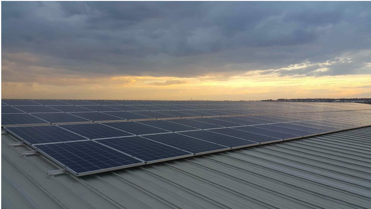
Figure 7.7. Example of Solar PV.
