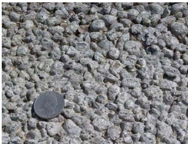
Figure 9.37. Example of pervious concrete pavement surface layer, with quarter to for scale. 404
