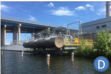
WE Energies Switchgear / Inlet Yards Excluded from overlay for safety
