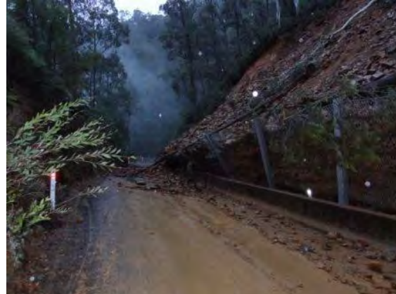
Road closure due to rock fall, 20kms east of Khancoban 22 July 2013.
