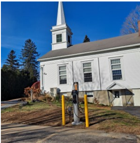
Wayne’s new EV Charging Station
