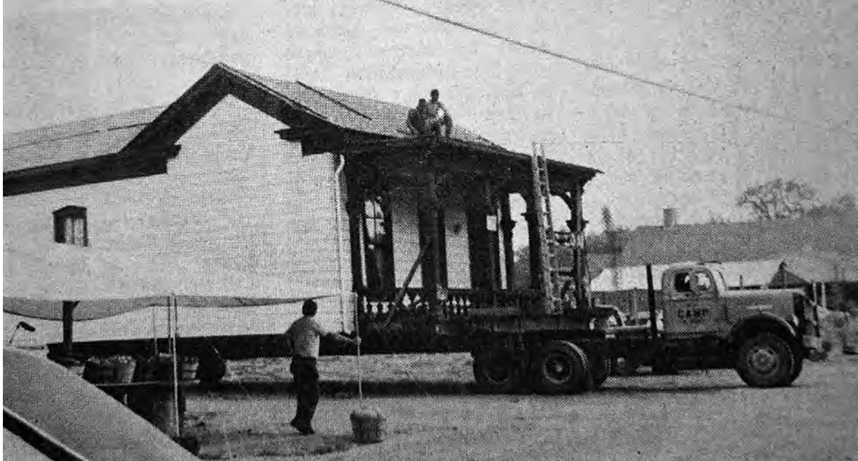
Moving day for the Malloy House which was relocated from East Main St. to New Highway 96 West.
