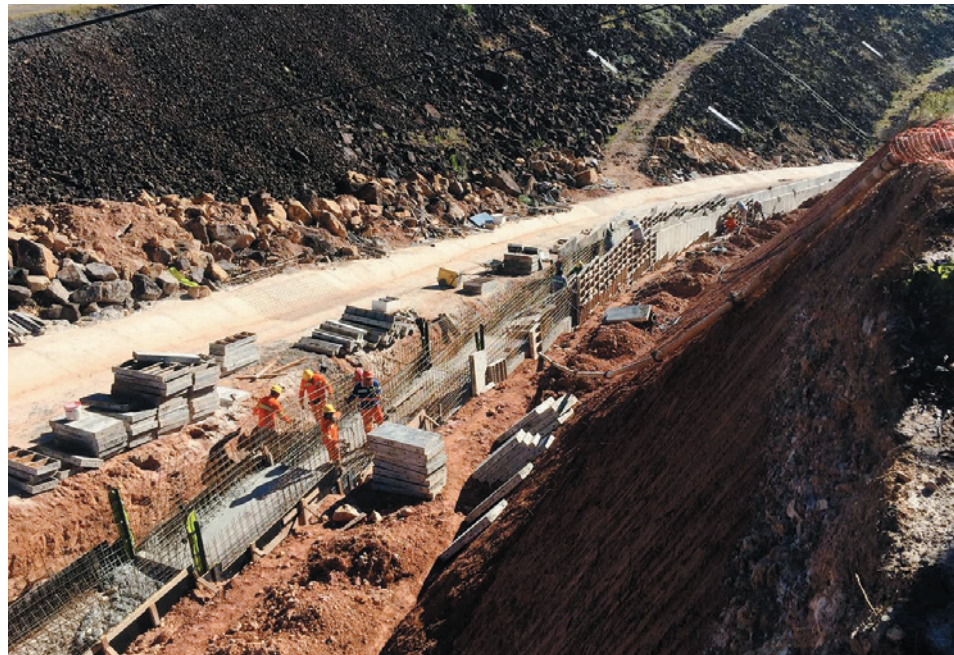
Construction work at the tailings dam of INB Caldas, May 2019 (Photo by Acervo INB)
