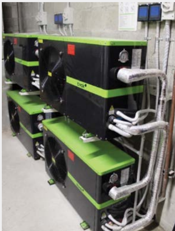
Figure 21 CNCC's heat pumps and storage tanks
