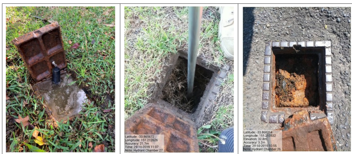
Figure 4.2: Examples of unsuitable chambers for logger installations.
