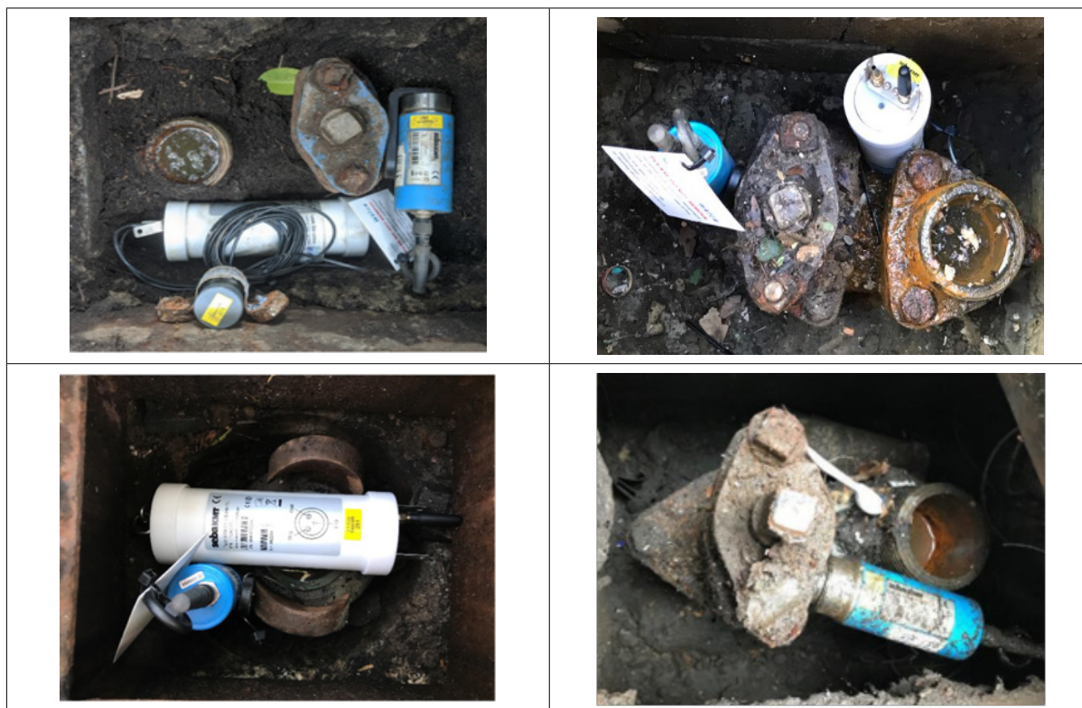
Figure 4.14: Log N-3 installations in Sydney CBD and Liverpool (right angle adapter top row, bottom left) and directly mounted to asset (bottom right).
