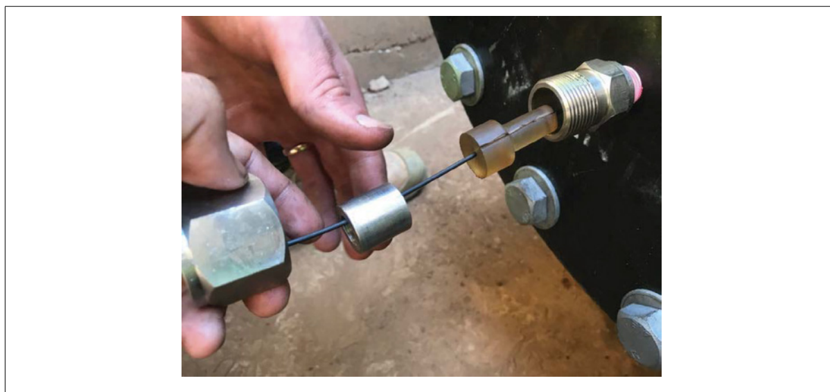
Figure 3.3: Sealing method around 2.15mm armoured tow cable. Conax cable gland used with polyurethane casting.
