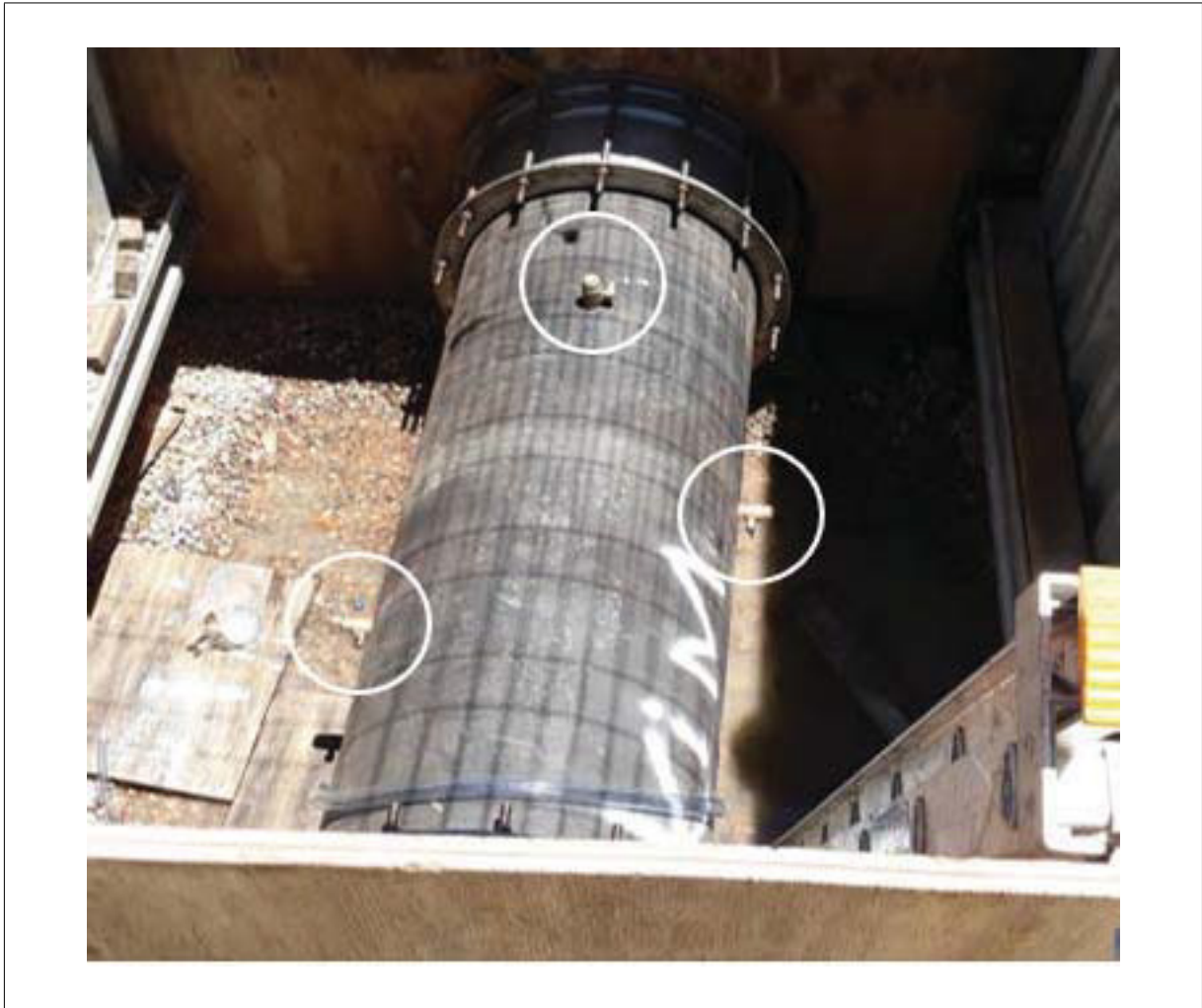
Figure 3.6: The simulated leak points were tapped into a pipe section at 3, 6, 9 and 12 o'clock around the pipe circumference. Three leak points visible and circled.
