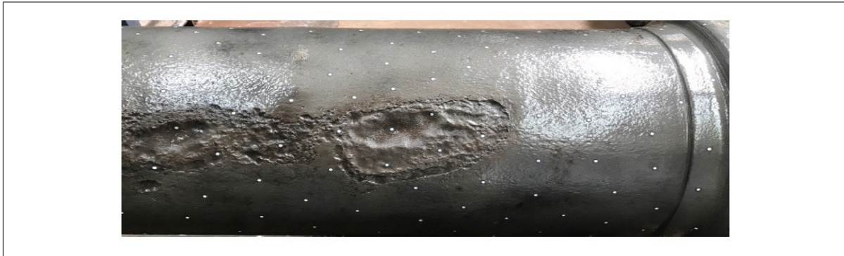
Figure 6.1: Example of localised corrosion along the bottom of a 100 year old cast iron pipe recovered from a Brisbane suburb (© RE Melchers).
