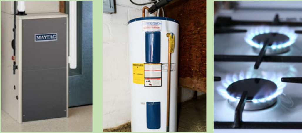
Fossil fuel technologies: furnace, gas hot water heater, gas range
