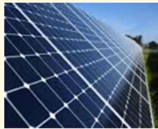
On-site Solar PV
