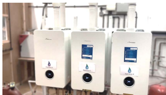
Demonstrated 180 kW six boiler cascade
