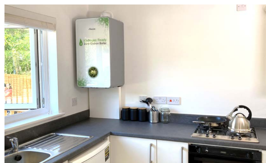
Hydrogen Home, Gateshead
