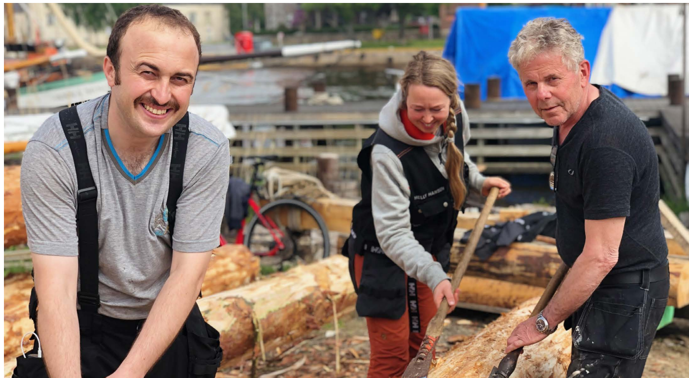
Volunteers have put in a total of nearly 3000 work hours on the Hope Cathedral in 2020.
