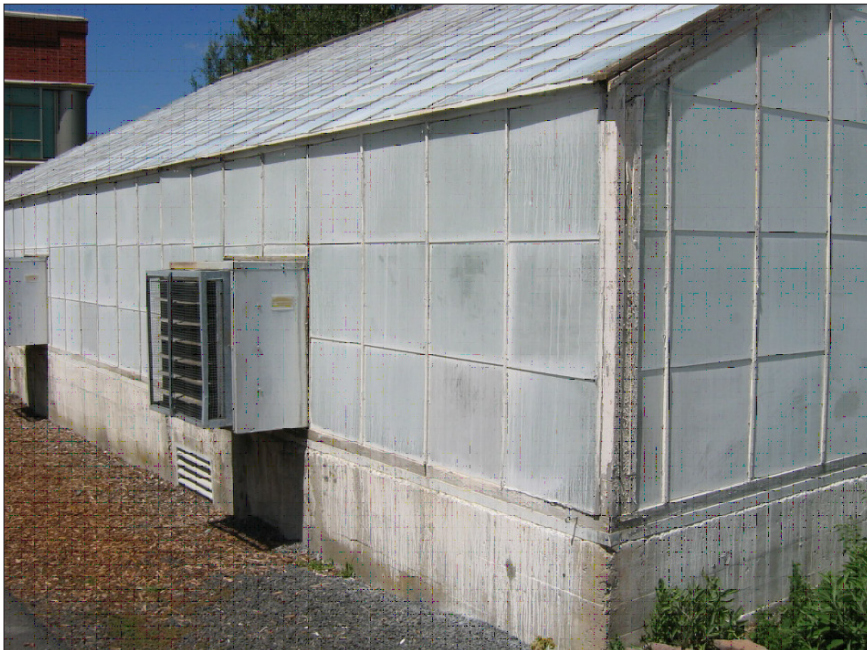
Figure 4. A mixture of white latex paint and water sprayed on a greenhouse structure will reduce the amount of light and heat penetrating through the glass.
