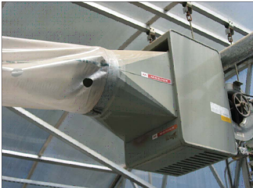
Figure 3. Forced air heater with an attached polyethylene tube to distribute warm air more uniformly throughout the greenhouse.
