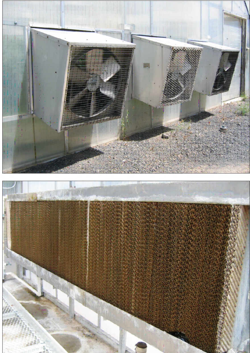
Figure 5. The fan system (top) and pad system (bottom) work together to ventilate and cool a greenhouse.
