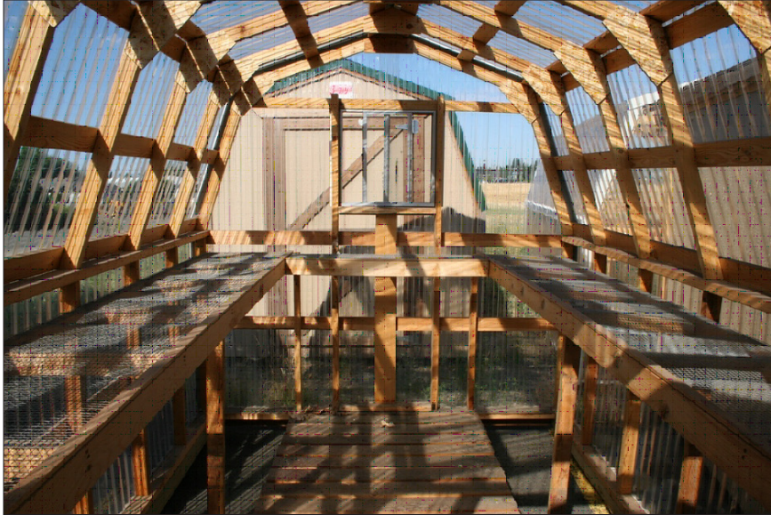
Figure 2. Wooden supports are used for the structure while wooden frames with wire mesh serve as workbenches in this hobby greenhouse.
