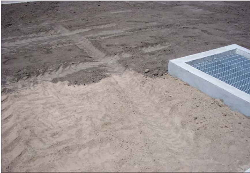
Figure 5. Topsoil layered over subsoil during final site grading and preparation for planting.
