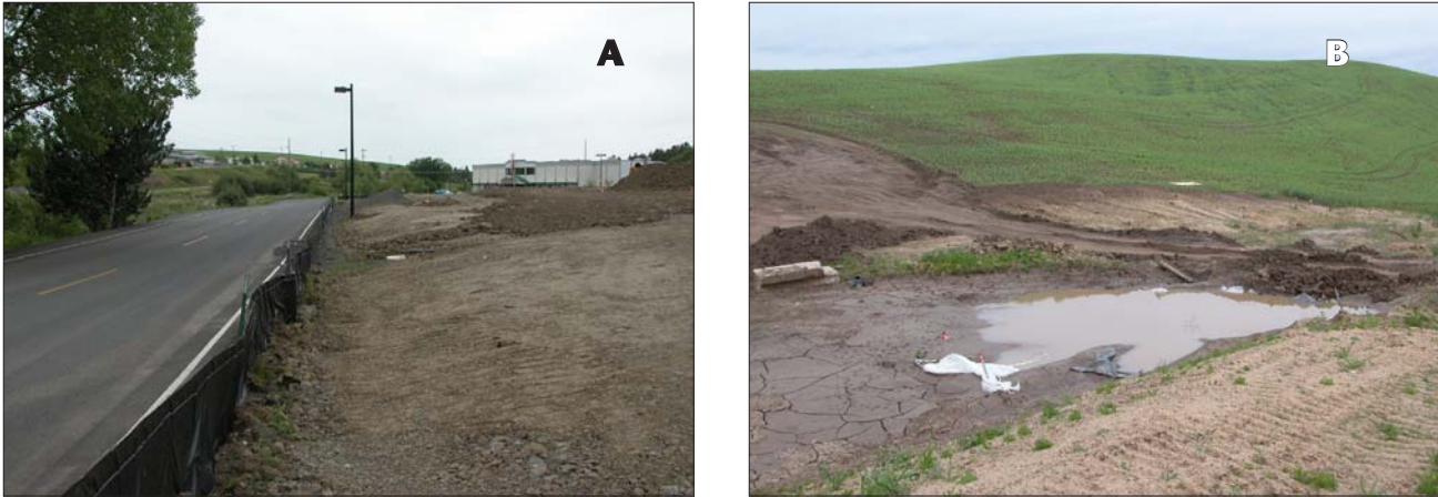
Figure 4. Common erosion control measures on construction sites: A) silt fence used to control gradual (sheet) runoff and erosion; B) sediment basin for retaining concentrated flow.
